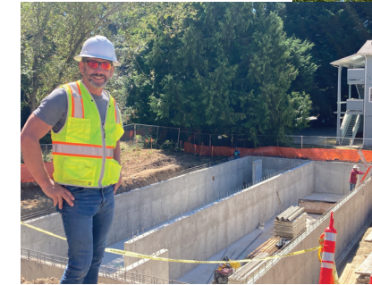
Pictured above Island Home. A detention vault at the Ericksen Community (left) will control stormwater.
